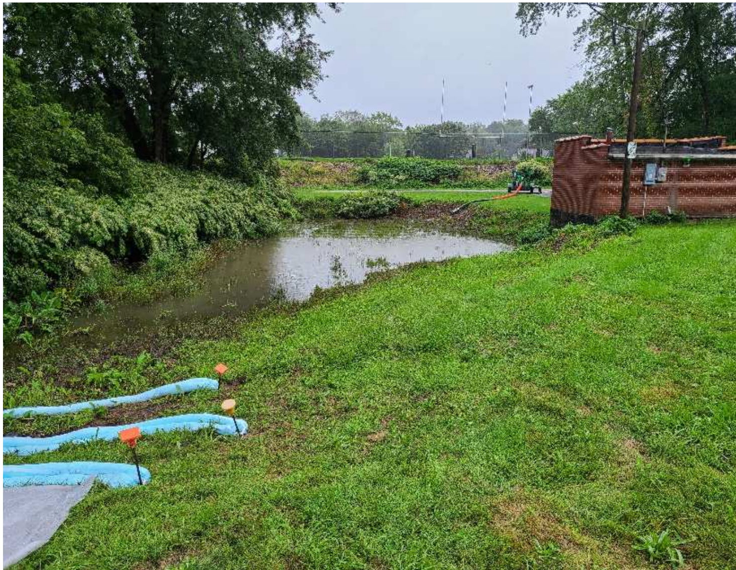
Merrifield Pump Station, 2pm
