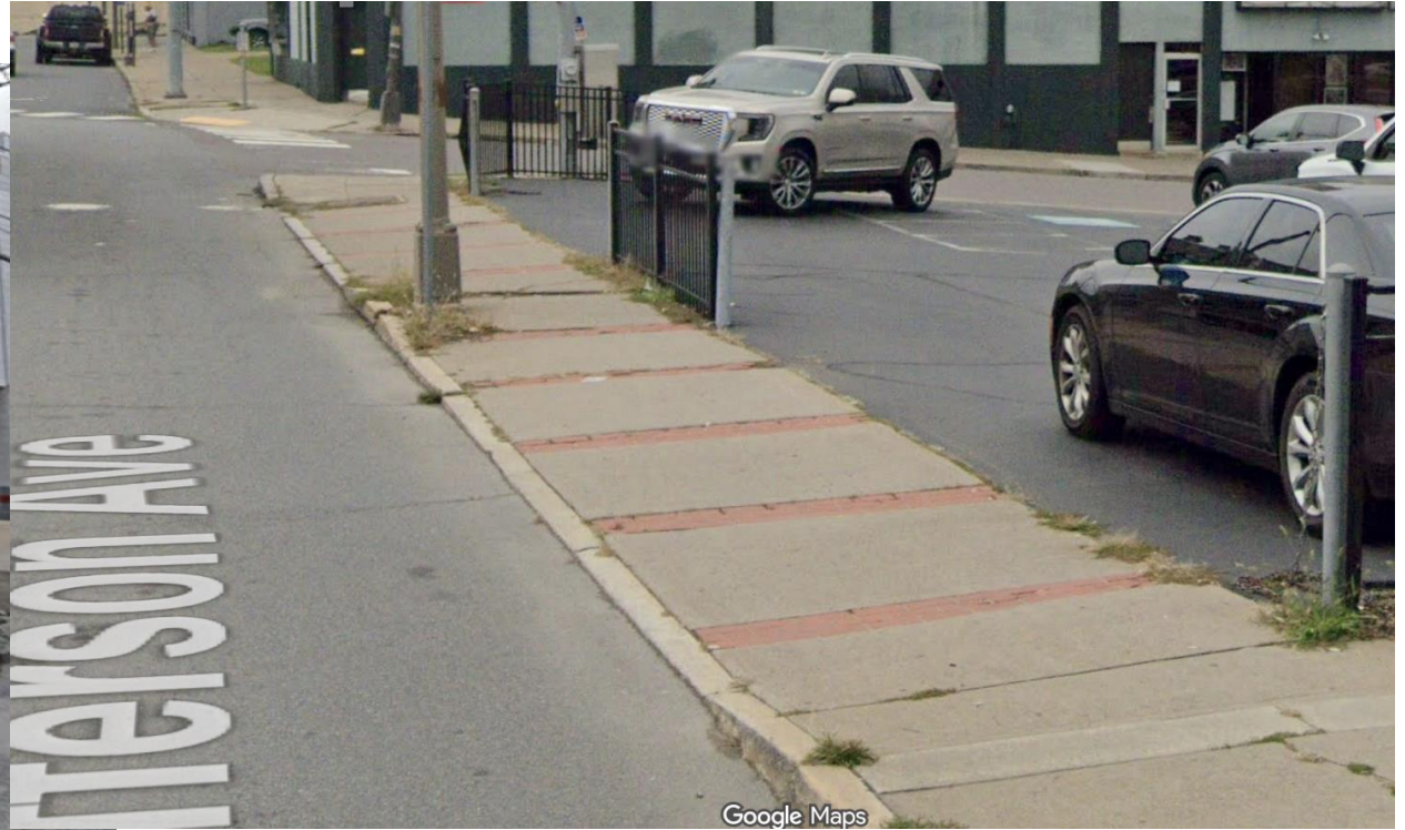
EXAMPLE: POOR SIDEWALK SURFACES: ADAMS AVE. (LEFT) JEFFERSON AT BIDEN (RIGHT)
